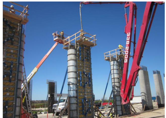
CCW is a $212-million highway funded by the federal and provincial governments. (Photo: SNC-Lavalin Group Inc.)
